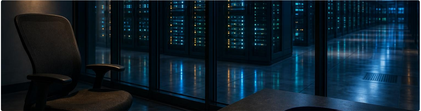
An empty chair and badge face glowing computer servers in a quiet, high-tech room.
