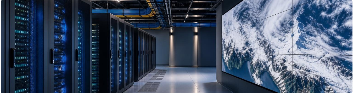
Rows of supercomputer cabinets sit beside a display of satellite-like weather patterns over mountains and ice.
