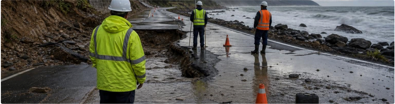
Workers inspect flood damage on a coastal road under cloudy skies.
